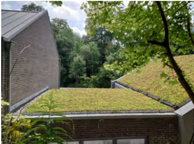
Green roofs supplementing blue-green infrastructure - This building has been designed with a sedum green roof which provides ecological benefits to the adjacent Water of Leith
