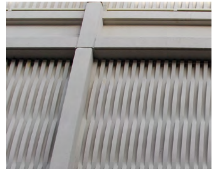
Textures created with concrete - Concrete panels with a textured surface treatment are used on this recent building on Princes Street.
